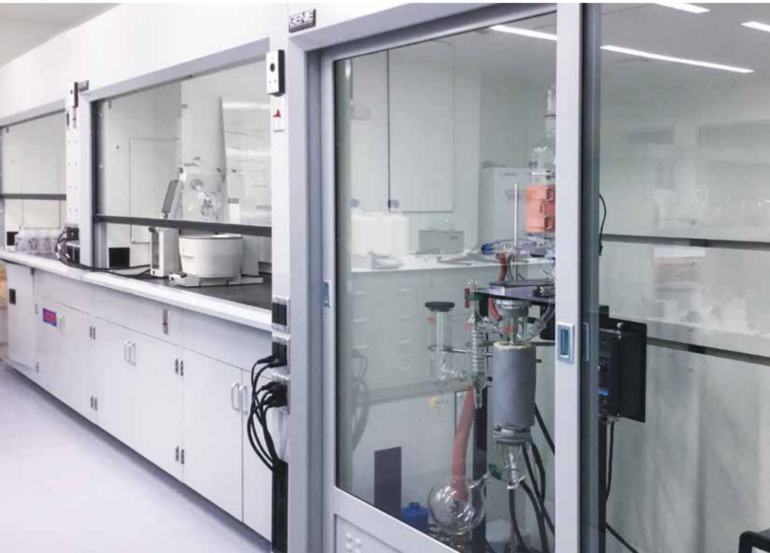
Exhaust hood made to fit client's apparatus.
